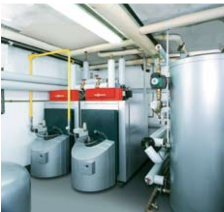
Vitoplex 300 installation in Audi Headquarters
