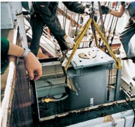
Vitoplex 100 installation on board the Gorch Fock Stralsund
